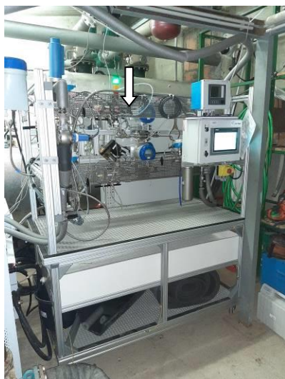
Figure 2a: First rack of the hardware twin in the field, with the injection point of the dosing pumps indicated by the white arrow.
