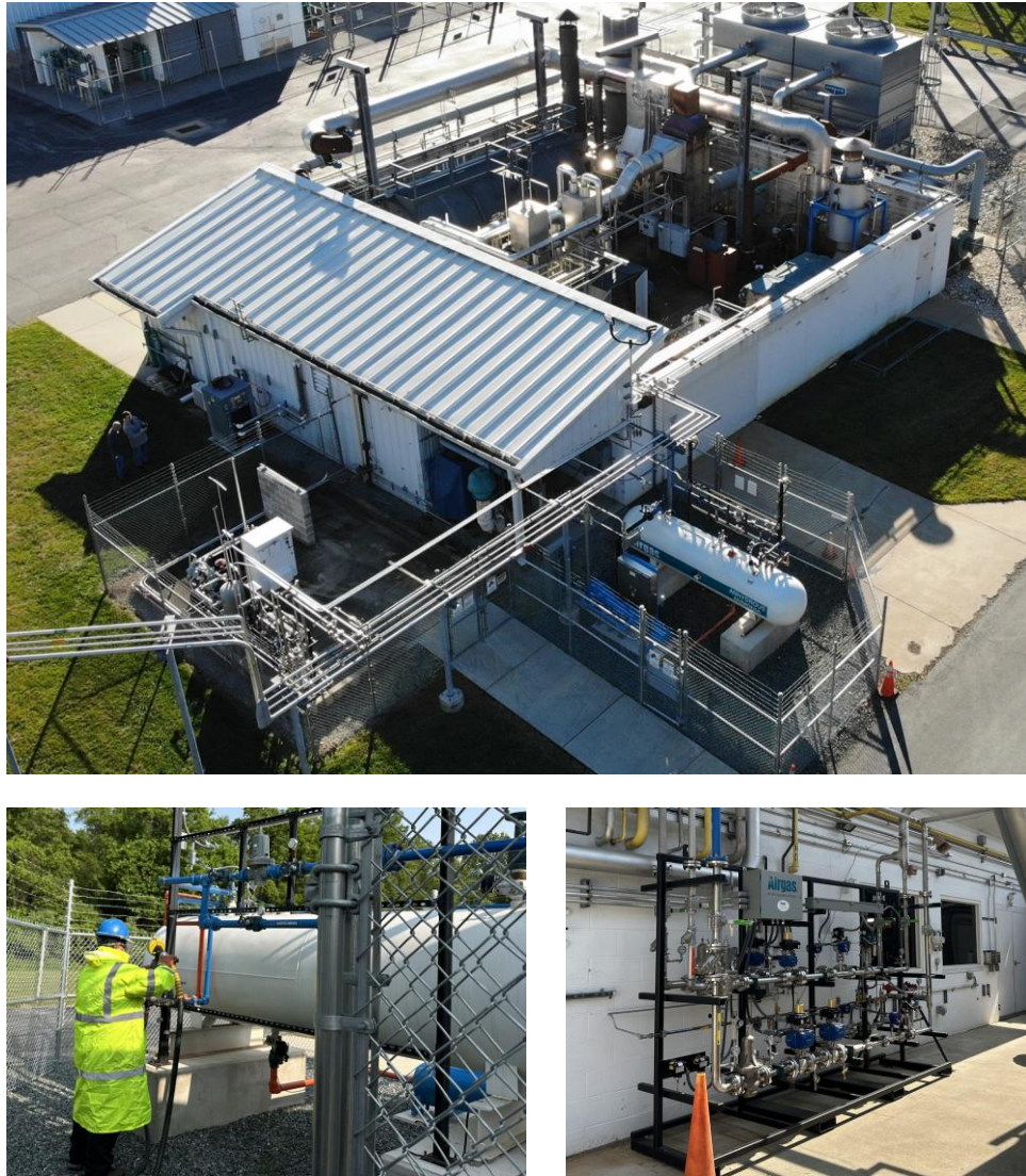
Figure 4: Combustion test platform with \text{NH}_3 combustion capability at Innovation Campus Delaware (top) with \text{NH}_3 tank (bottom left) and \text{NH}_3 flow control skid (bottom right).
