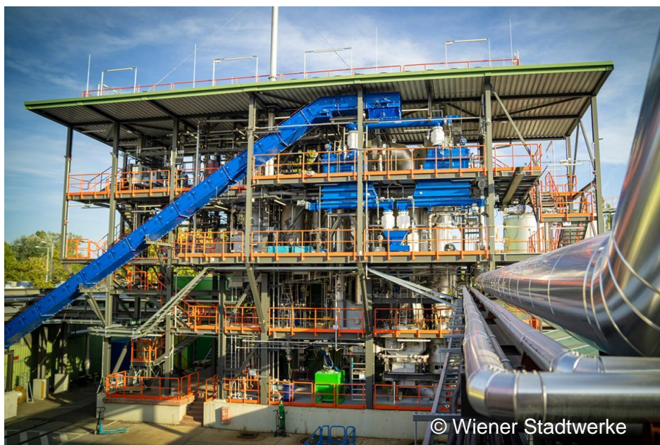
Figure 3: Syngas Platform Vienna at Wien Energie's site Simmeringer Haide.
